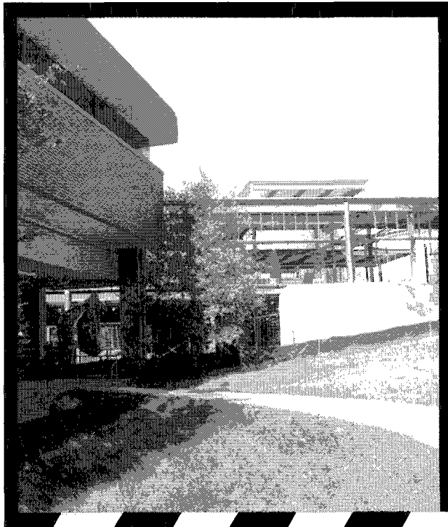
THE ADDITION TO THE LAW SCHOOL, NOW UNDER CONSTRUCTION, WILL ADD 58,000 MUCH-NEEDED SQUARE FEET TO THE BUILDING, GIVING THE SCHOOL NEARLY 160,000 SQUARE FEET OF SPACE.
